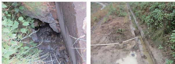
图 10 坡脚、平台水沟地下水出露 Fig. 10 The underground water emergence from slope foot, platform ditch
